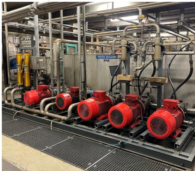
Figure 13: Hydraulic system for cooling and bearing lubrication as part of the Nipco-Roll
